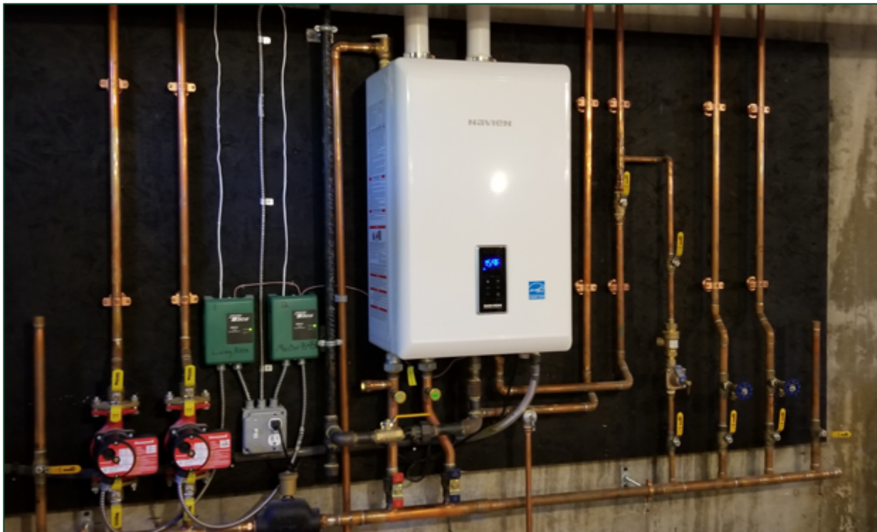
Figure 71. Two Heating Zones with Two Honeywell Zone Valves
