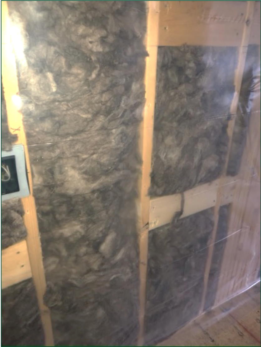
Figure 48. Rater's Photograph Showing Insulation Around Electrical Box and Framing
