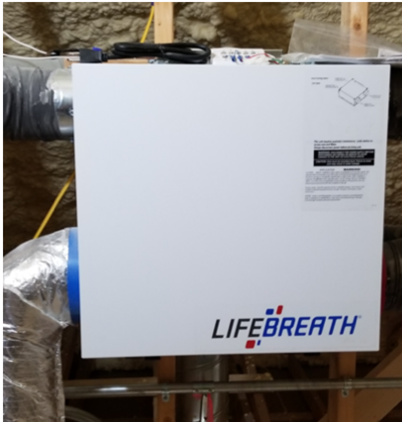
Figure 73. Heat Recovery Ventilation System Observed by a Rater
