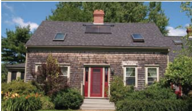
Solar Thermal System on houses in Rockport (top) and Lincolnville (bottom), both installed by ReVision Energy
