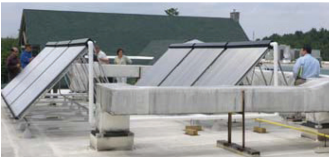
Solar thermal water system at L.L.Bean funded by a Commercial Project Grant
