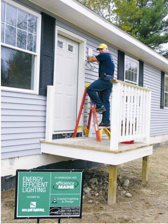
Electrician Dave Gerrish donates his time installing ENERGY STAR® lighting at Habitat for Humanity's Naples, Maine project
