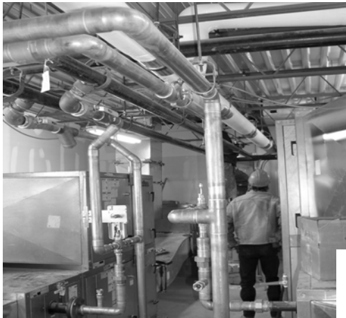
High efficiency HVAC equipment installed in Congin
