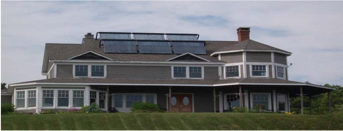
Installation by Revision Energy Rockport
