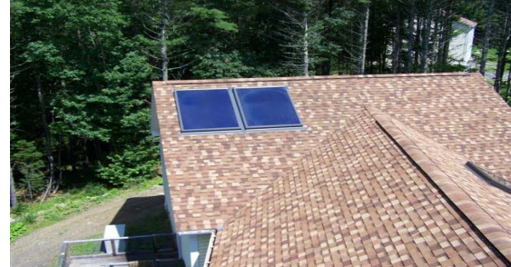
Installation by Mid Coast Energy Systems
