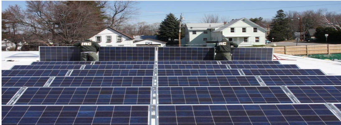
Installed by IRC Group, Augusta
