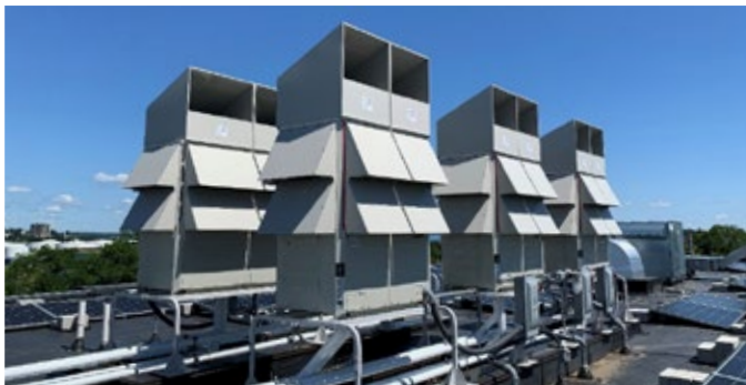
VRF equipment at Betsy Ross Crossing
