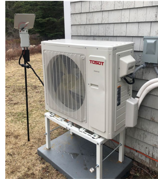
Outdoor Unit & Meter
