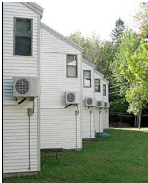
Figure 6: Multifamily heat pump installation.
