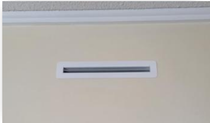
An inlet vent for a transfer fan.
