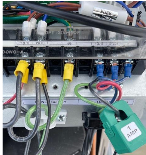
Figure 15. 1A CT Placed on Wire Powering Indoor Fan
