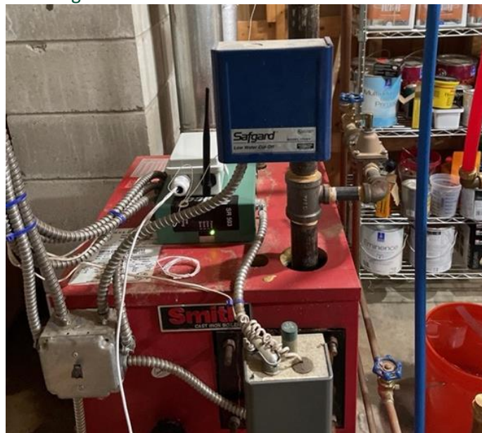
Figure 17. Cell Phone Meter on a Smith Boiler
