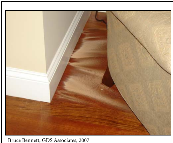
Figure 11. Construction Dust Displaying Air Infiltration
