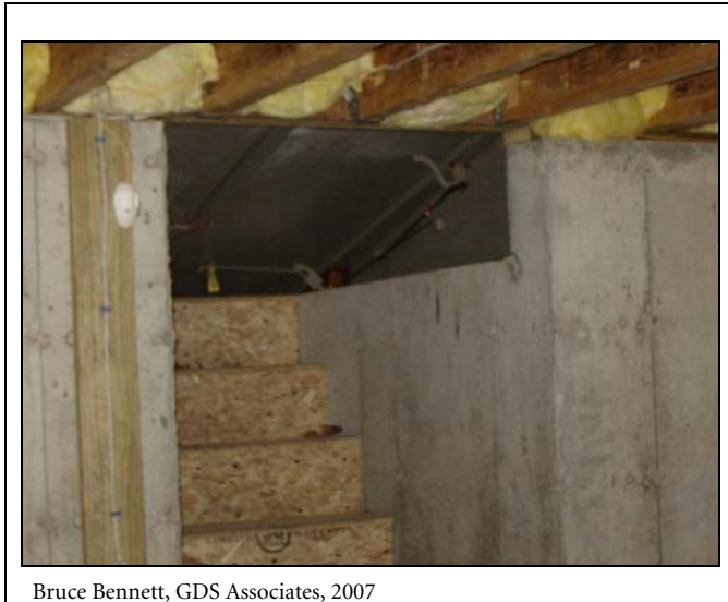
Figure 5. Uninsulated Foundation Walls.
