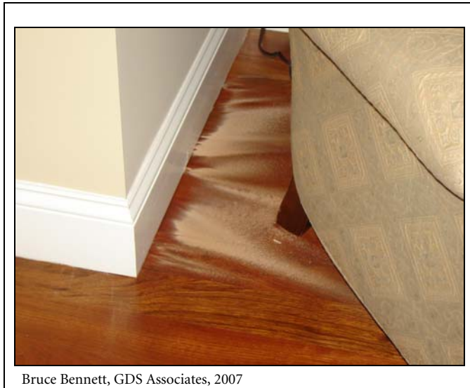
Figure 11. Construction Dust Displaying Air Infiltration
