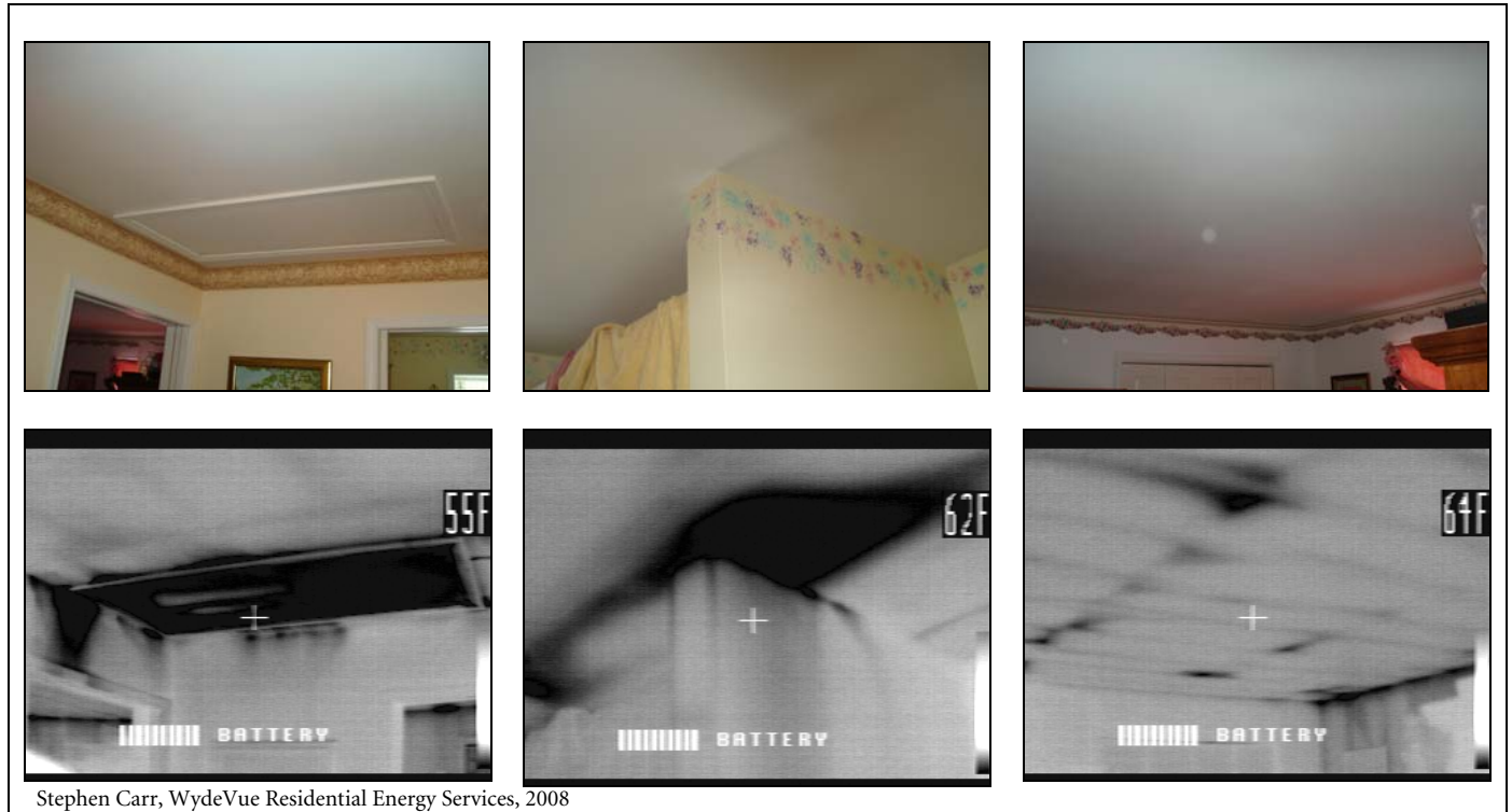
Figure 6. Typical Gaps in Ceiling Insulation
