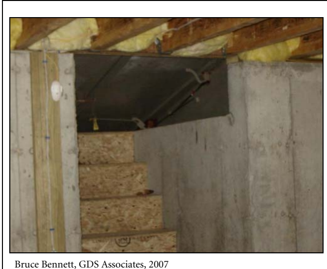
Figure 5. Uninsulated Foundation Walls.
