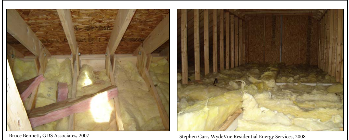
Figure 7. Typical Haphazard Ceiling Insulation Installation
