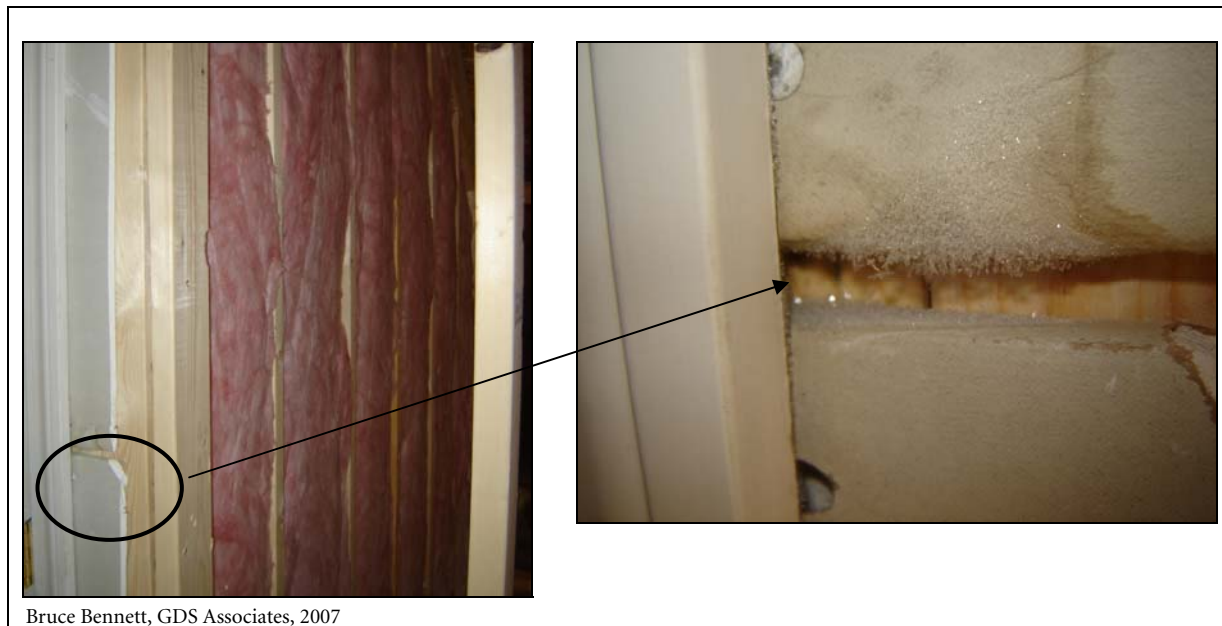
Figure 10. Effects of Poor Air Sealing
